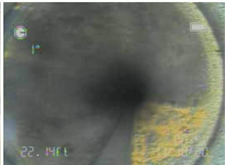
Figure 2 – Replaced Black Steel Pipe (2020 Assessment) In an adjacent section where galvanised mains were replaced with black steel and nitrogen protection was applied, observation of the piping shows only minimal corrosion. Six years later, the piping remains in good condition, demonstrating the effectiveness of nitrogen protection.
