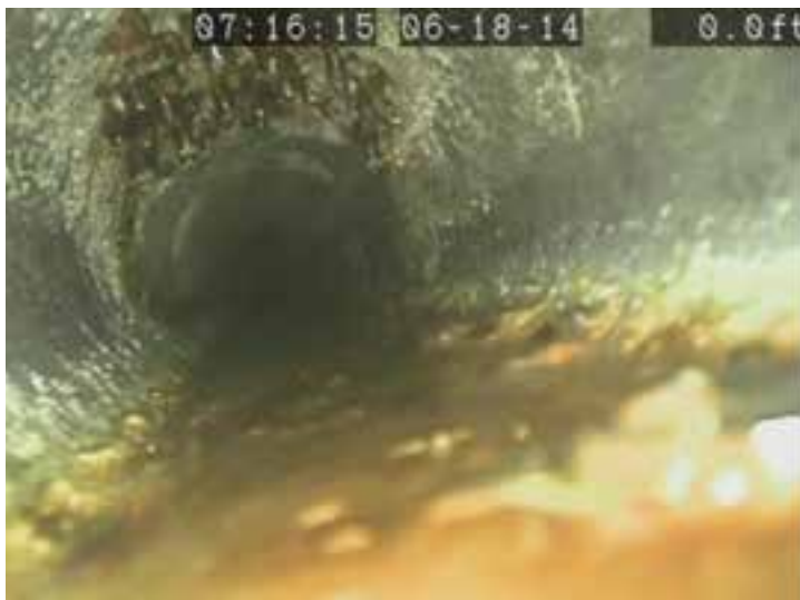
Figure 1 – Original Galvanised Main (2014 Assessment) Initial observation of the galvanised mains revealed severe corrosion damage, with large iron-oxide deposits and pitting underneath. These conditions led to multiple leaks within just a few years of operation.
