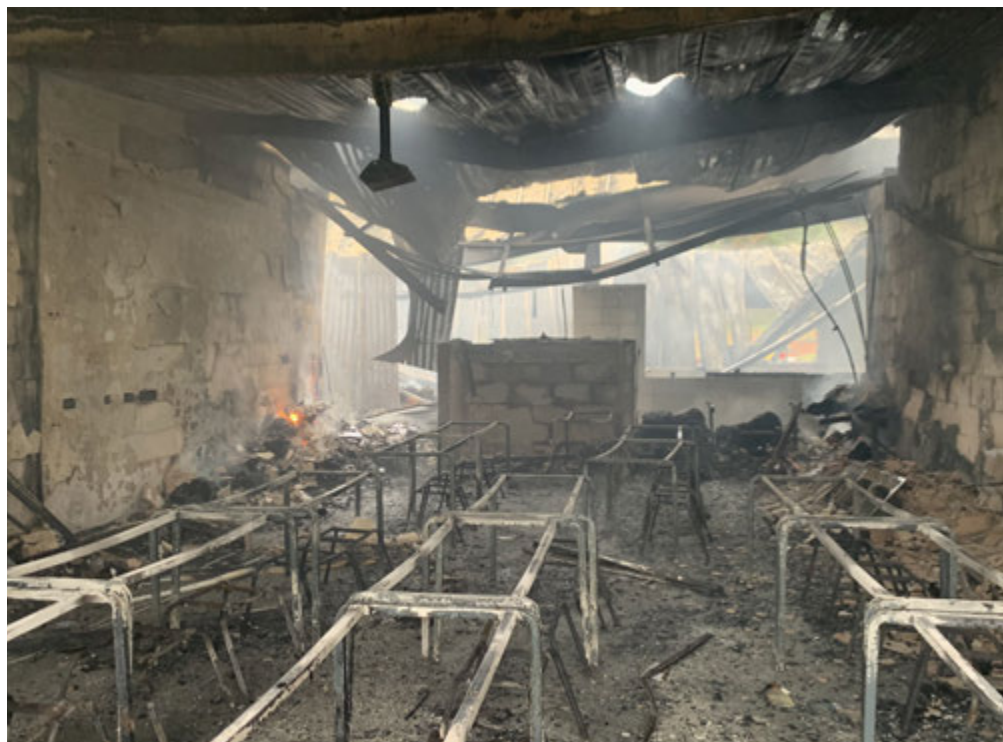
Greater Manchester FRS confirmed that three sprinkler heads prevented a fire in a college preventing fire spread.
